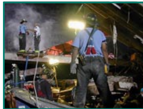
Even as night fell firefighters and rescuers worked the debris piles.
